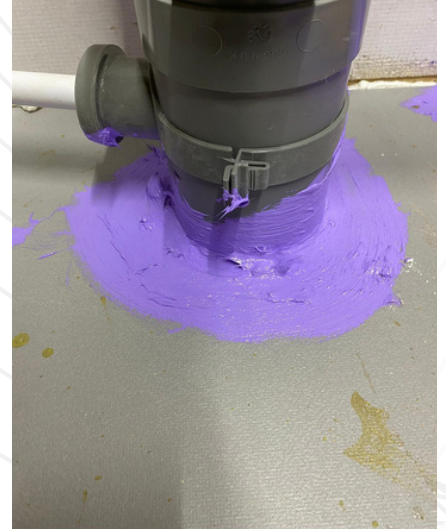
5.1.4 Soil stack through floor
