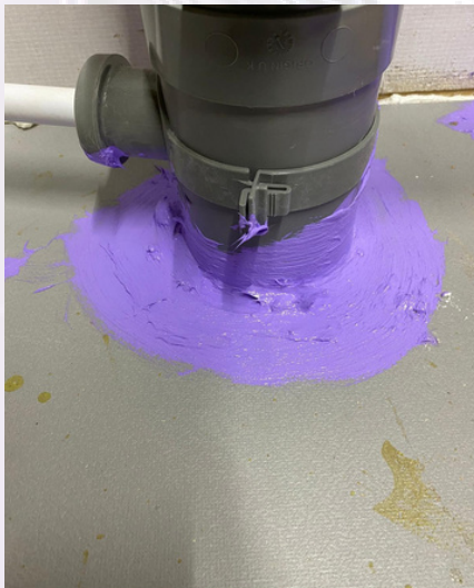
Soil stack through floor
